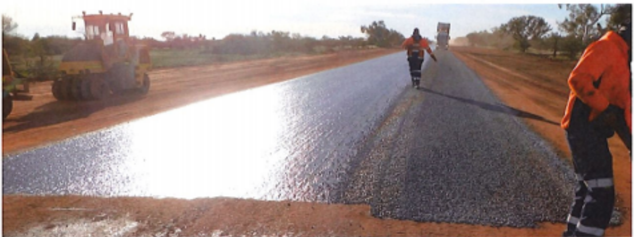
Dalgely Downs - Landor Rd SLK 76.89 - 002.JPG - Sealing First coat of 14mm stone.
