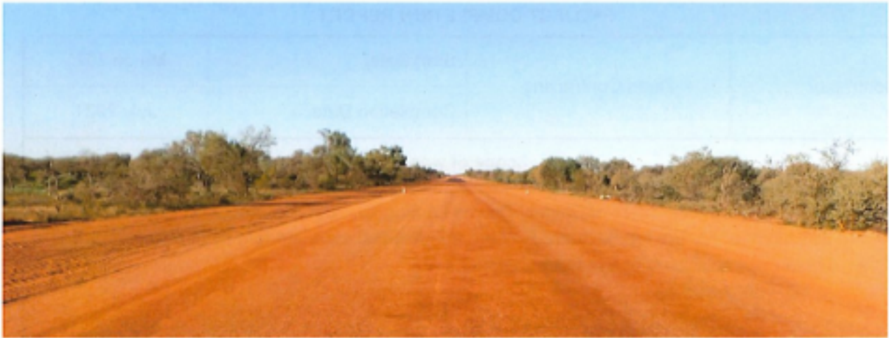
Dalgely Downs - Landor Rd SLK 71.39 - 001.JPG - Photo showing area prepared ready for sealing.
