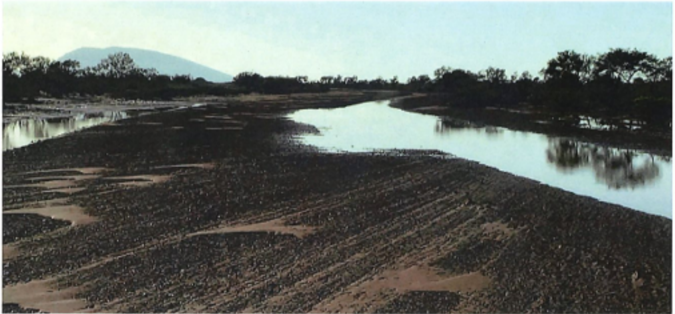
Cobra Mt Augustus Rd Silc 30.25 - Defect
