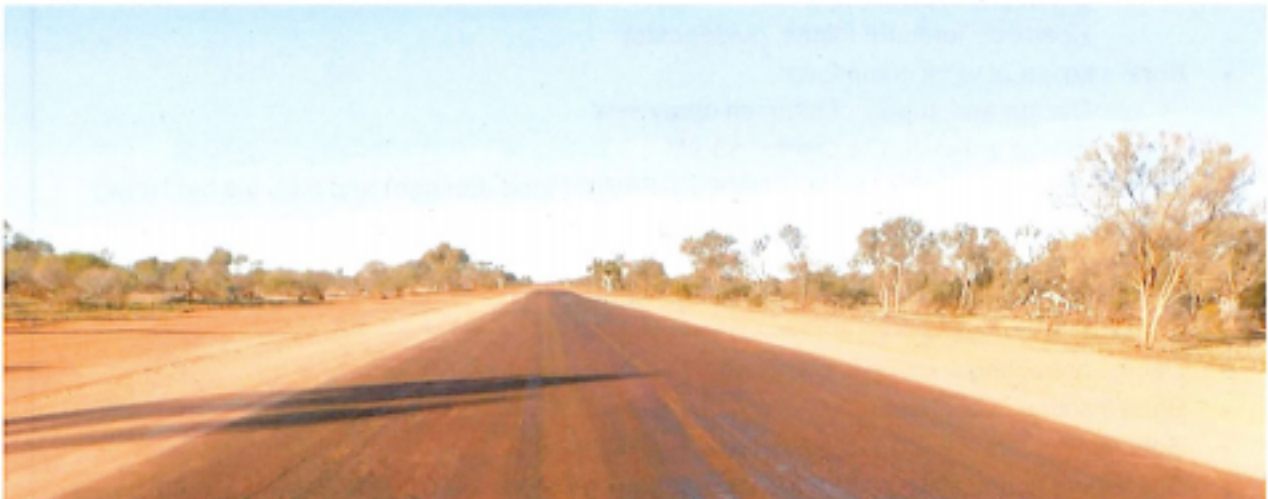
Dalgely Downs - Landor Rd SLK 73.87 - 001.JPG - Photo showing Prime seal in floodway.
