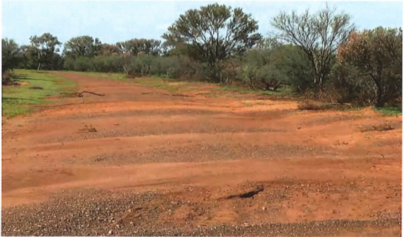
Bingegaroo Rd S1k 3.00- Defect.
