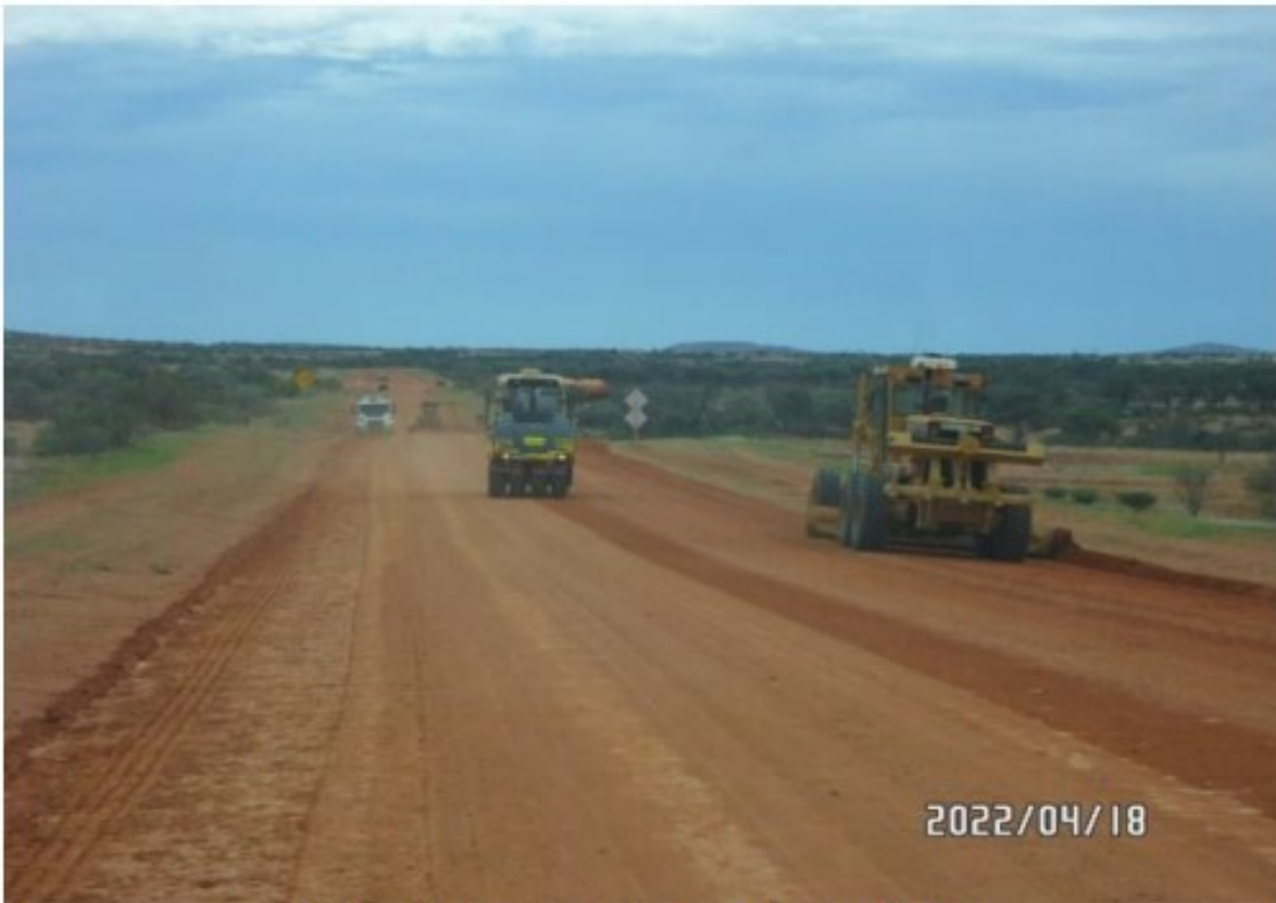
Cobra Dairy Creek Rd – from previous April report
