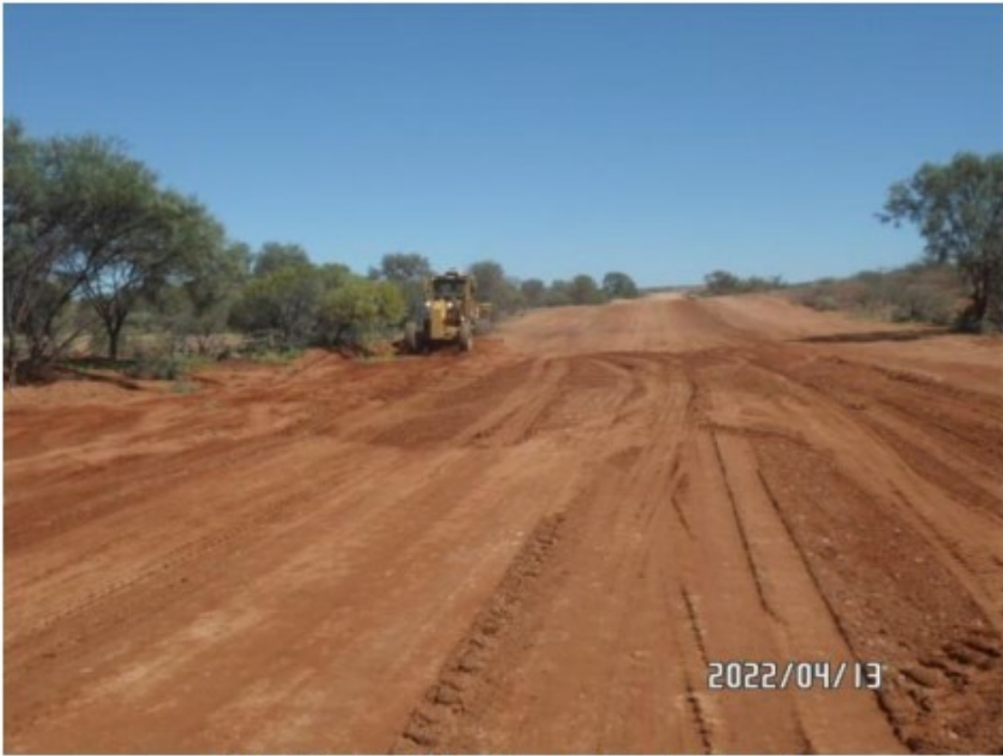
Cobra Dairy Creek Rd – from previous April report
