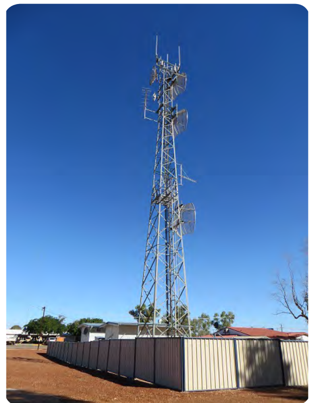
Gascoyne Junction Telstra tower
