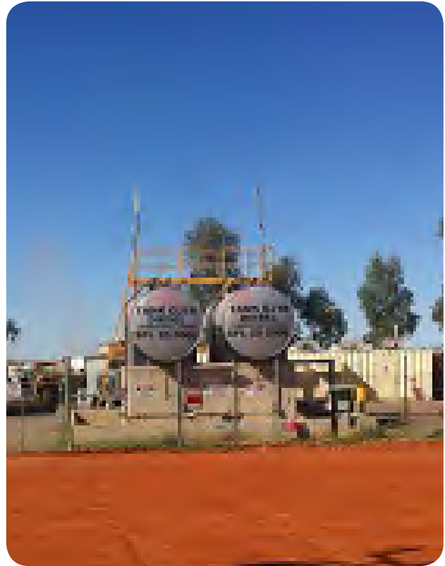
Gascoyne Junction power station
