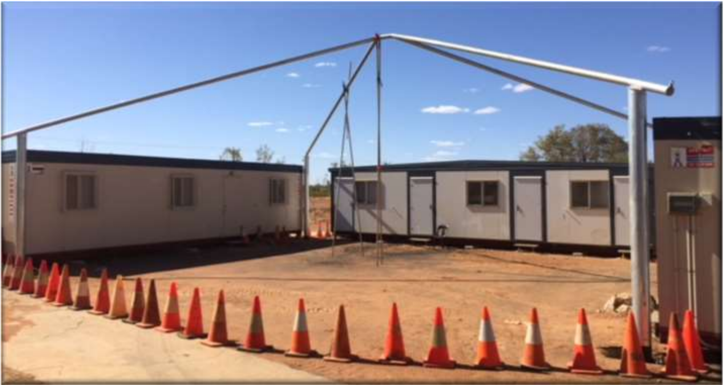
The new shade structure at the Donga's behind the Pavilion, which will be much appreciated by the Local Community during the sweltering Summer Months.
