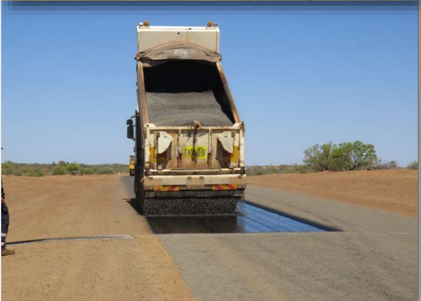
End Tipper laying out the blue metal over the newly sprayed road surface.
