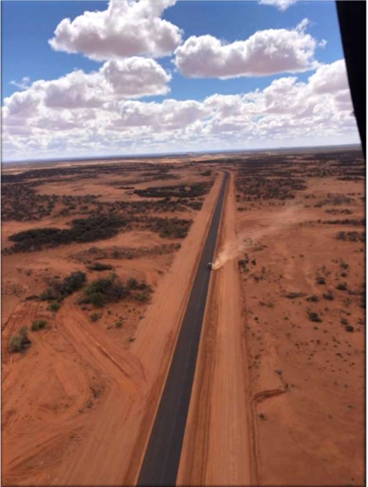
6.25km of new bitumen works situated 30kms east of Gascoyne Junction on the Carnarvon Mullewa Road.
